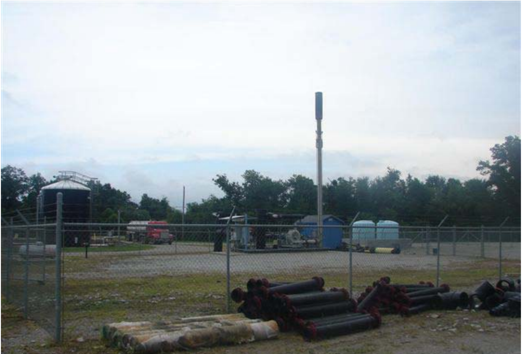
#2 Landfill Gas Flare with Leachate Collection Tank
